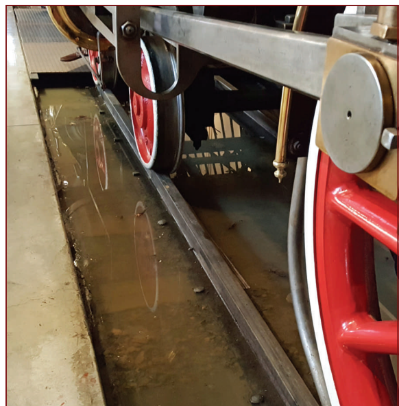
Flood waters percolated through ballast in the JIC.
