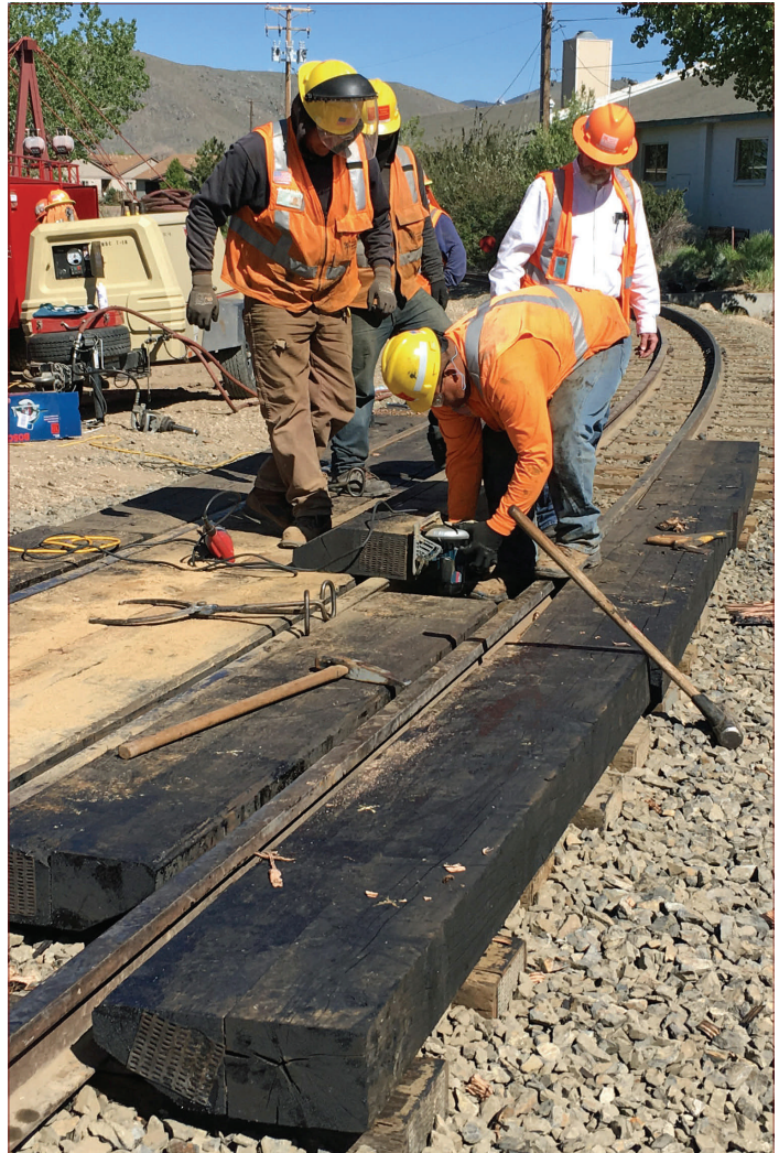
Track crews from Mountain States Contractors repair the grade crossing on the emergency access road, May 2017.
